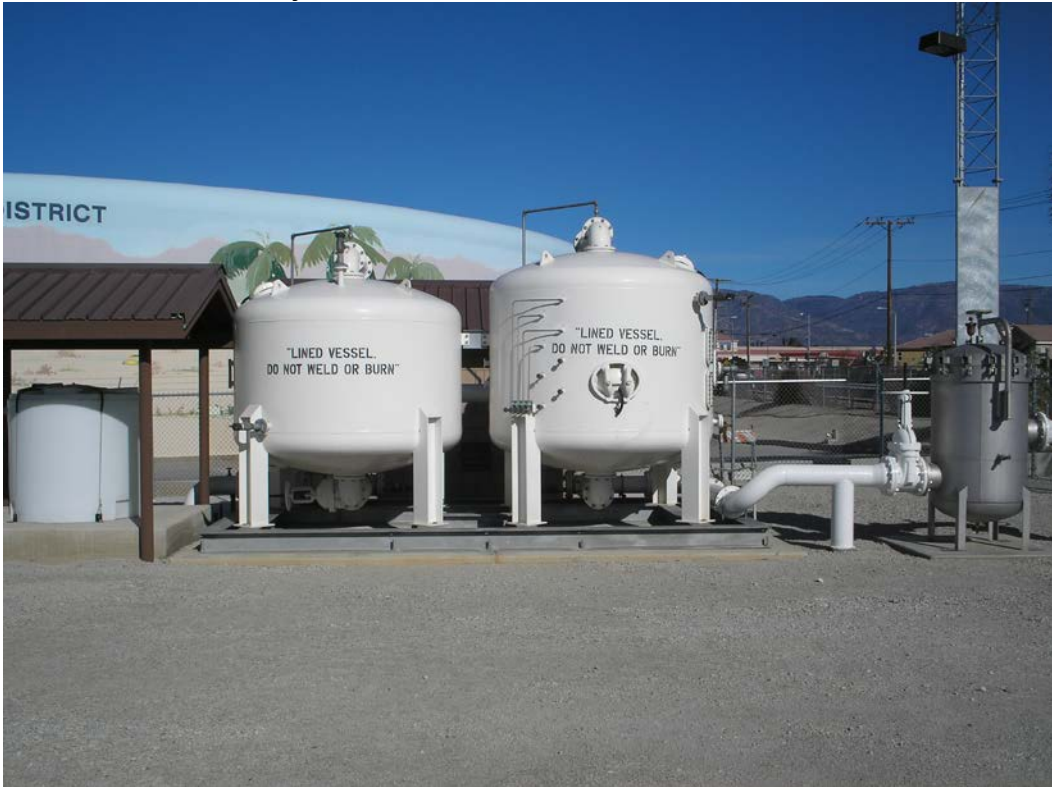
Figure 9. West Valley Water District (WVWD) Well # 11.
