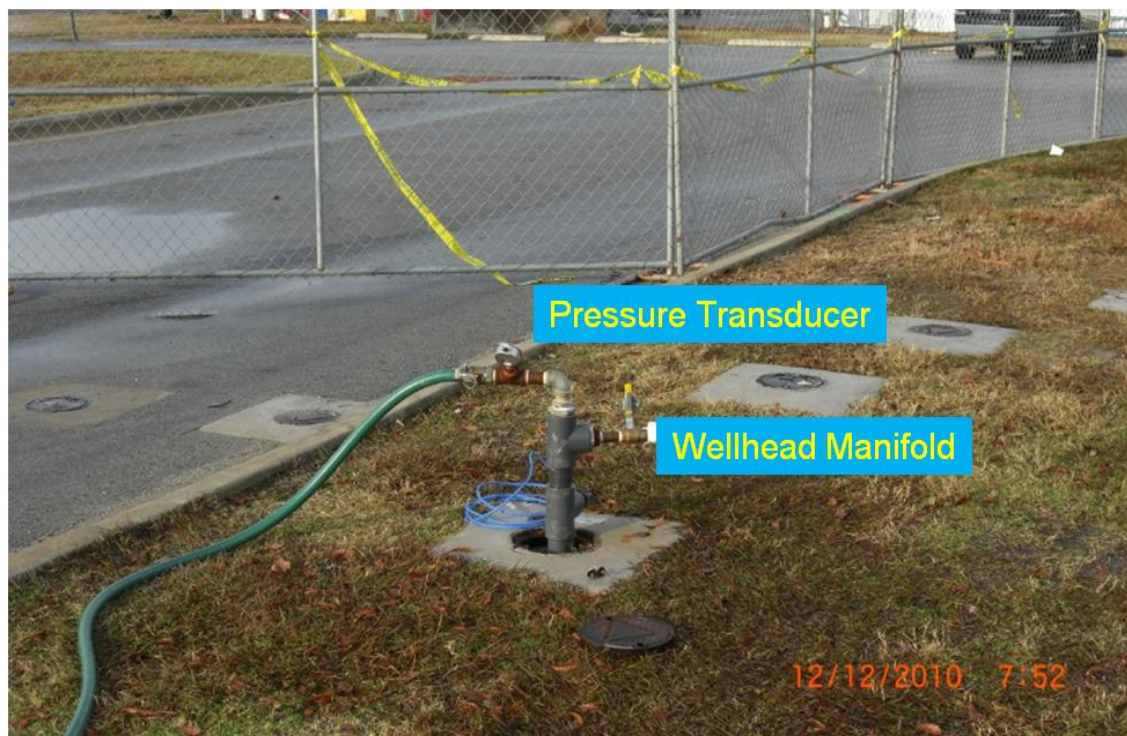
Figure 5-16. Injection wellhead manifold and pressure monitoring.
