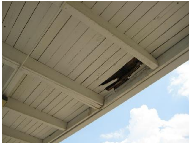
Figure 3 Building 515 Rotten Section
