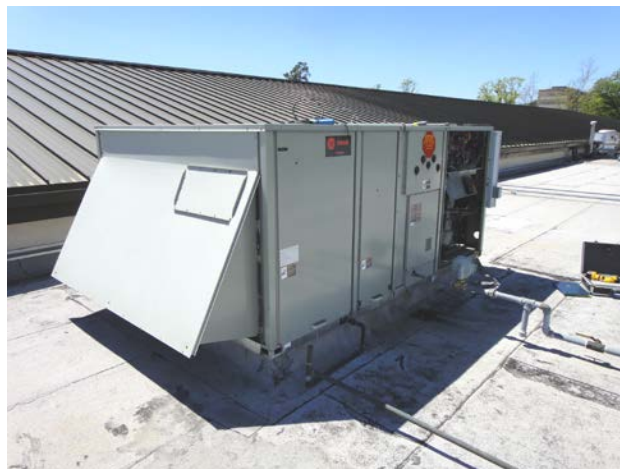
Figure 1 RTU-2 on roof of MCASB 1283.
