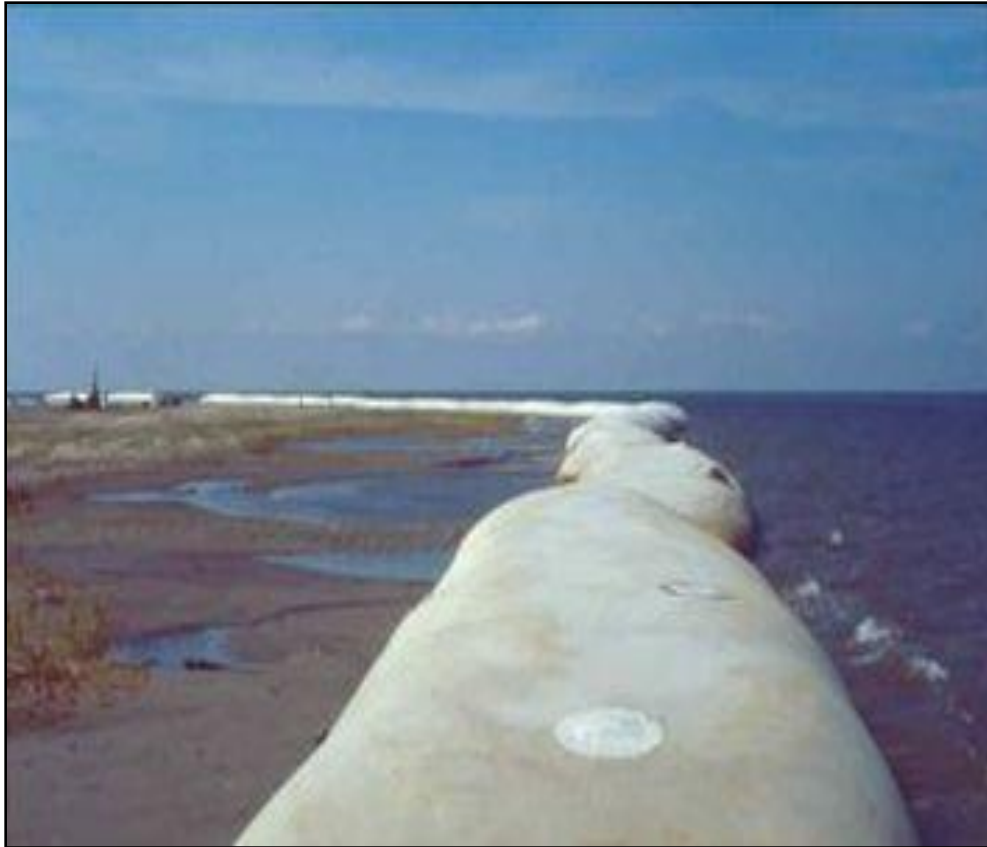
Figure 4. Geotextile tubes after dredged material had been placed behind them, western side of Barren Island (photo 2000).
