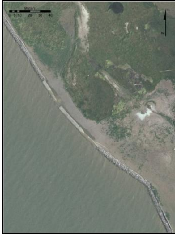
Figure 10. Western side of Barren Island where geotextile tubes were installed and failed (photo August 2005).
