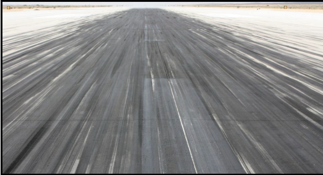
Figure 19. Runway 22L contaminated with rubber deposits prior to testing.
