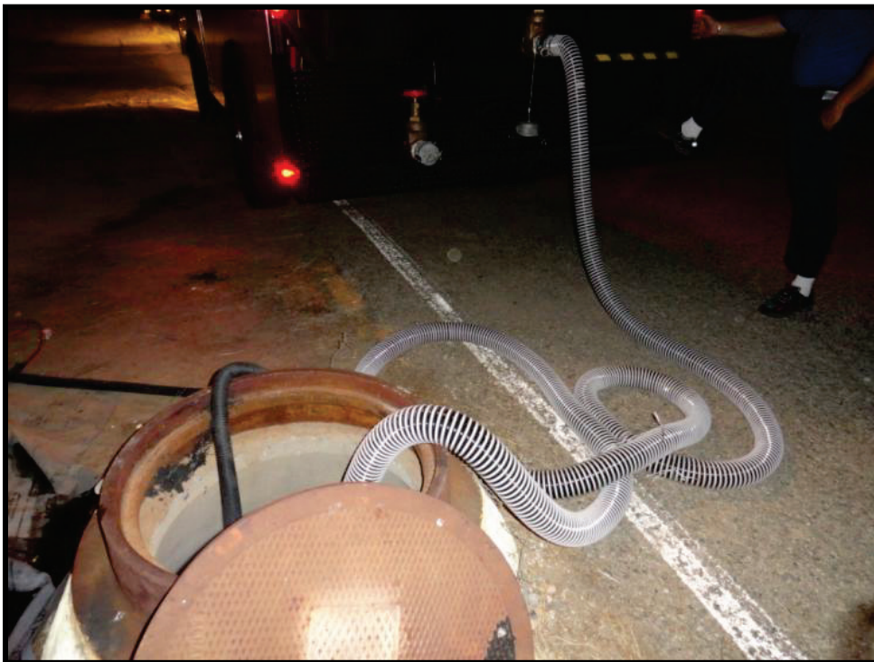
Figure 69. Cyclone 4006 gray water discharge.
