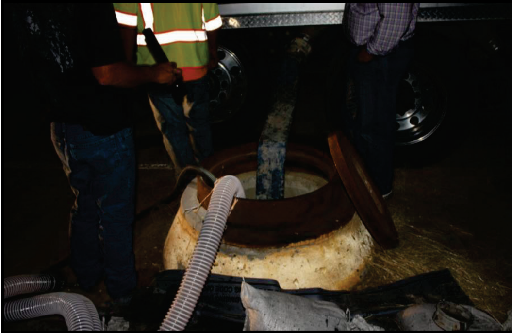
Figure 77. SH8000R gray water discharge.
