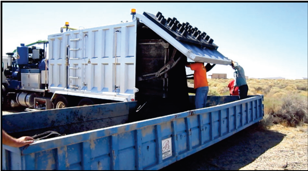
Figure 78. SH8000R dumps solids.
