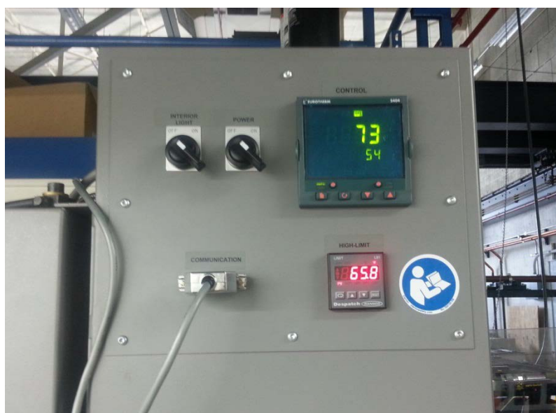
Figure G-15 Environmental Chamber Electrical Box with Communication Port
