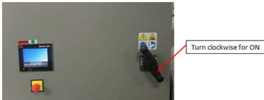
Figure C-6 Control Panel on Hydraulic Pump System
