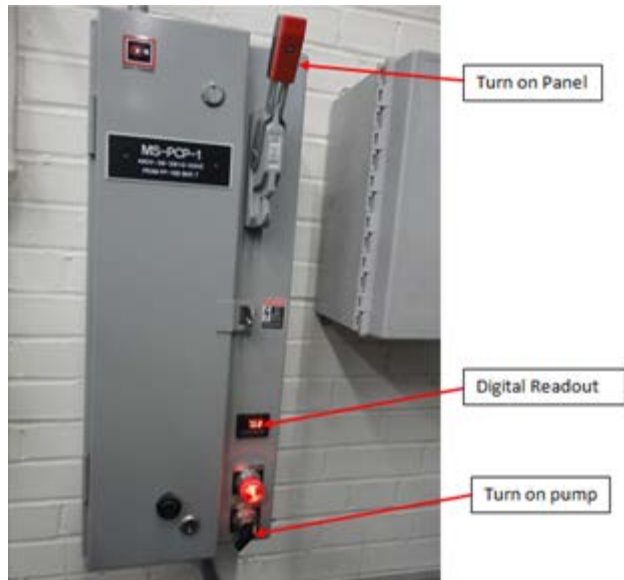
Figure C-2 Water Pump Breaker
