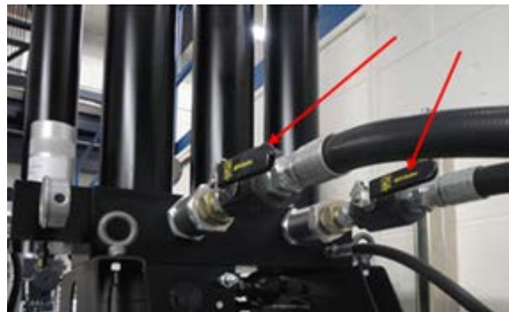
Figure C-3 HSM Supply and Return Valves
