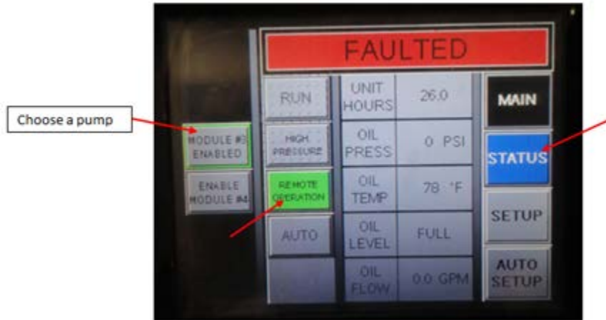
Figure C-8 Control Screen on Hydraulic Pump System
