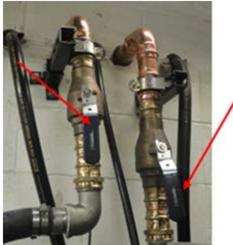
Figure C-5 Water Valves at Pump System
