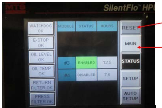
Figure C-9 Control Screen on Hydraulic Pump System
