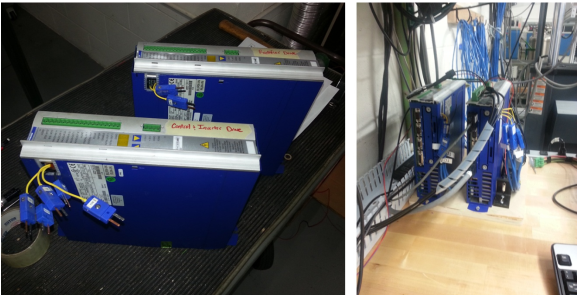
Figure F-7 Servodrive System Completed with Thermocouples
