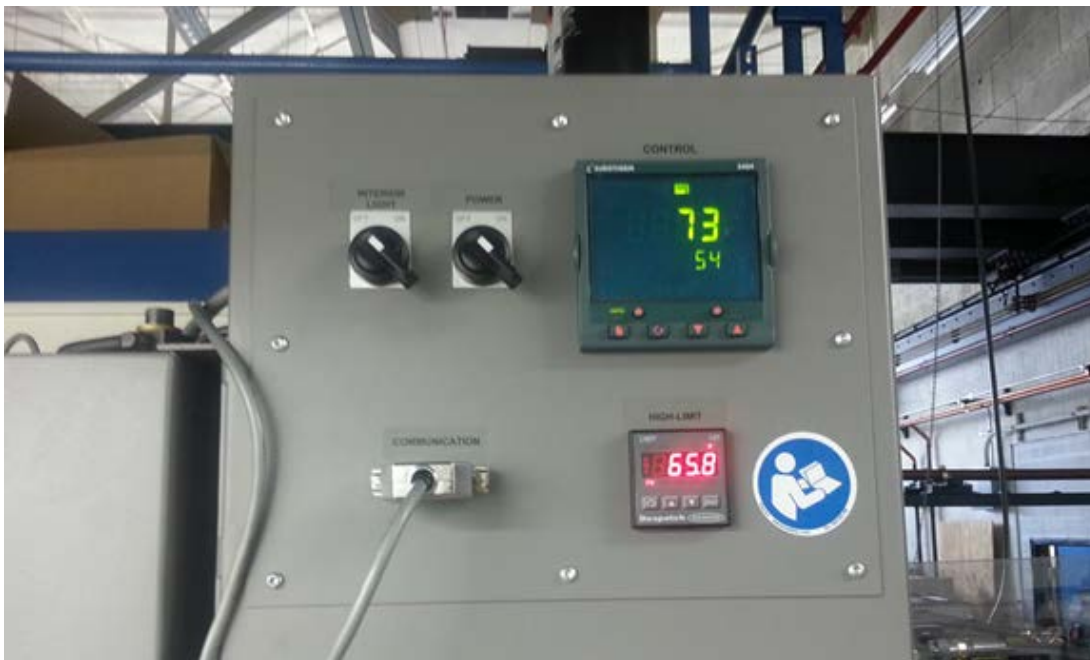
Figure C-23 Environmental Chamber Panel
