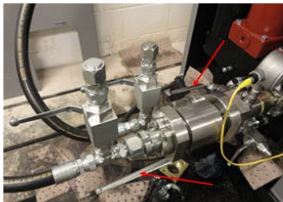
Figure C-4 HPU Supply and Return Valves
