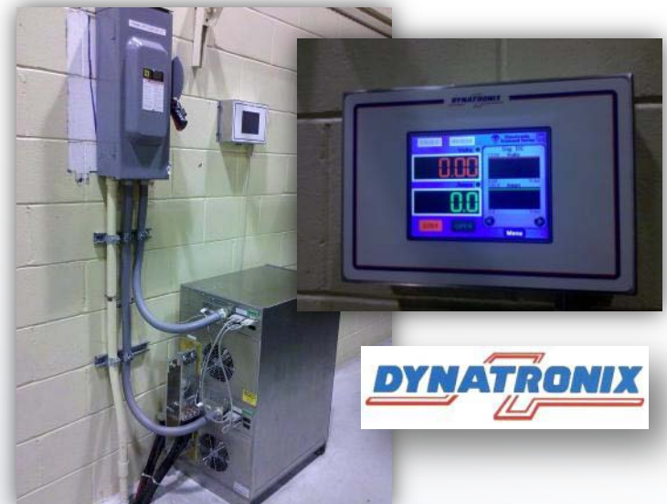
Activation Tank Power Supply
