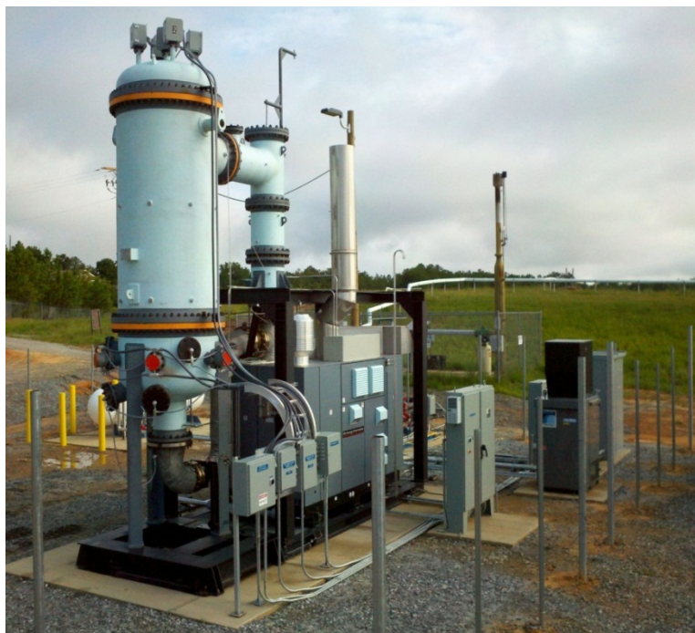
Figure 2. FP250 installed at 1 st Division Road landfill.
