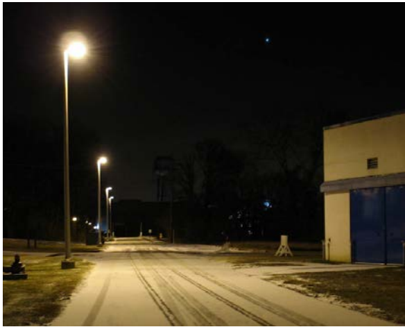
Existing HPS Lamps
