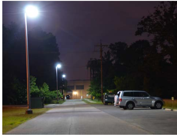
Newly Installed LED Street Lighting System
