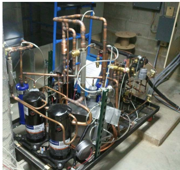
Figure 8. Mechanical housing installed at CAJMTTC.
