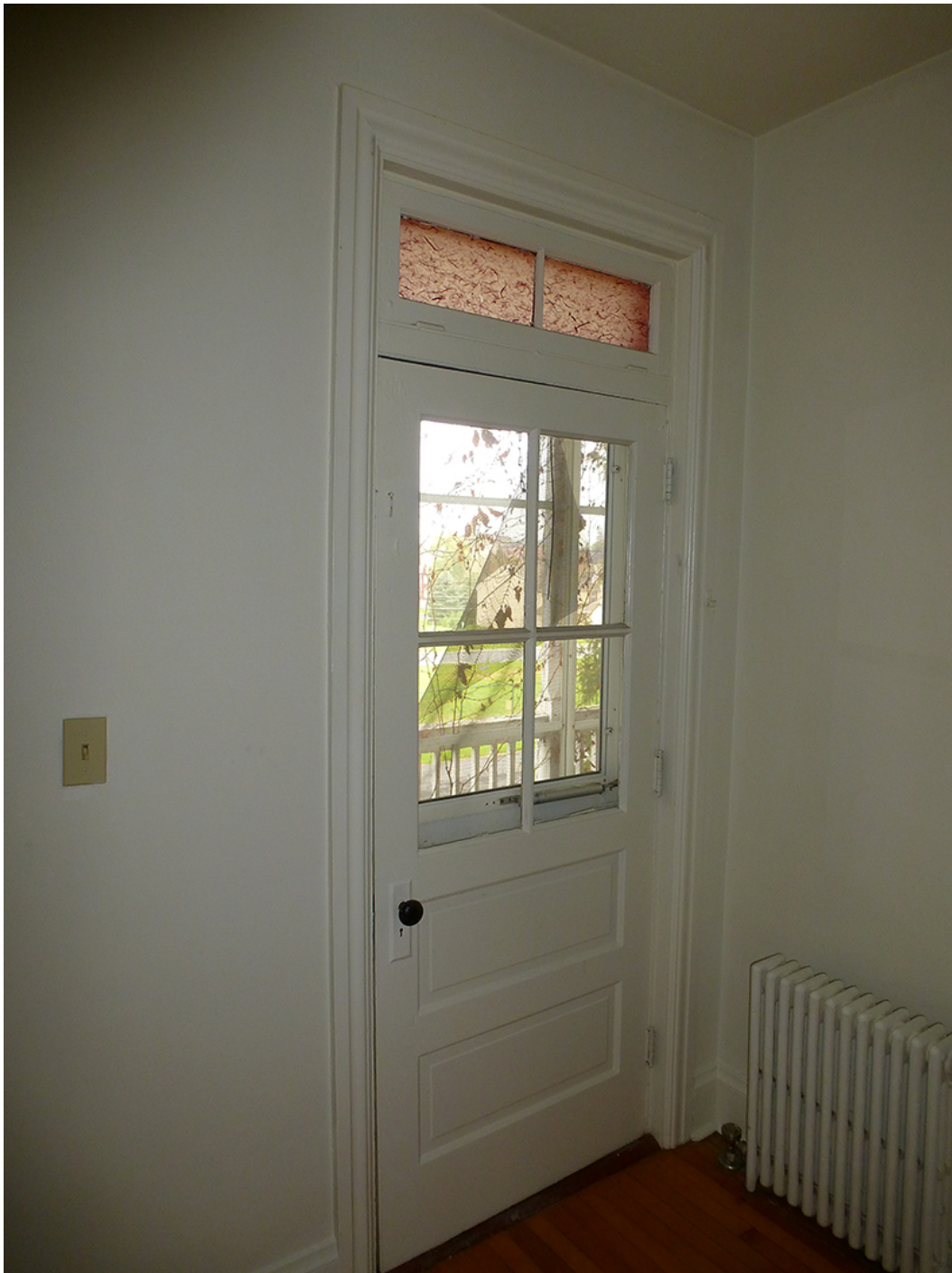
Figure 44. Door from the hallway in the ell to the east porch (ERDC-CERL, 2012).
