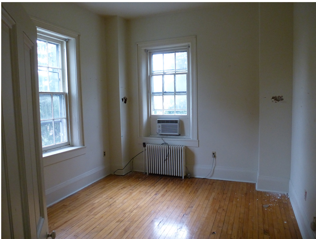
Figure 28. One of the two, small, second-floor bedrooms in the south part of duplex (ERDC-CERL, 2012).
