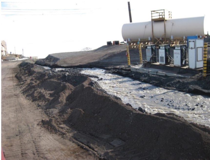
Figure 7. Side berm emplaced as a temporary solution to contain the runoff during an extreme event, 19 December 2010 (photo by Lynette Barna, CRREL).
