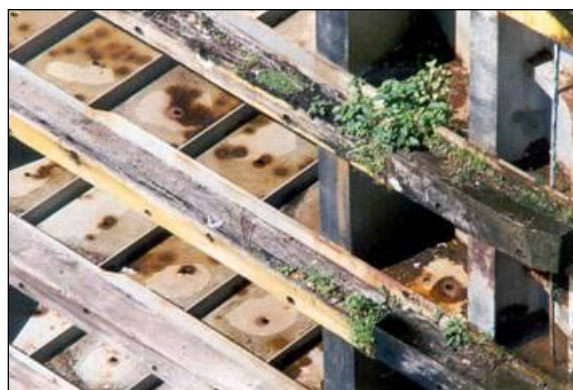
Figure 7. Corrosion on a miter gate.
