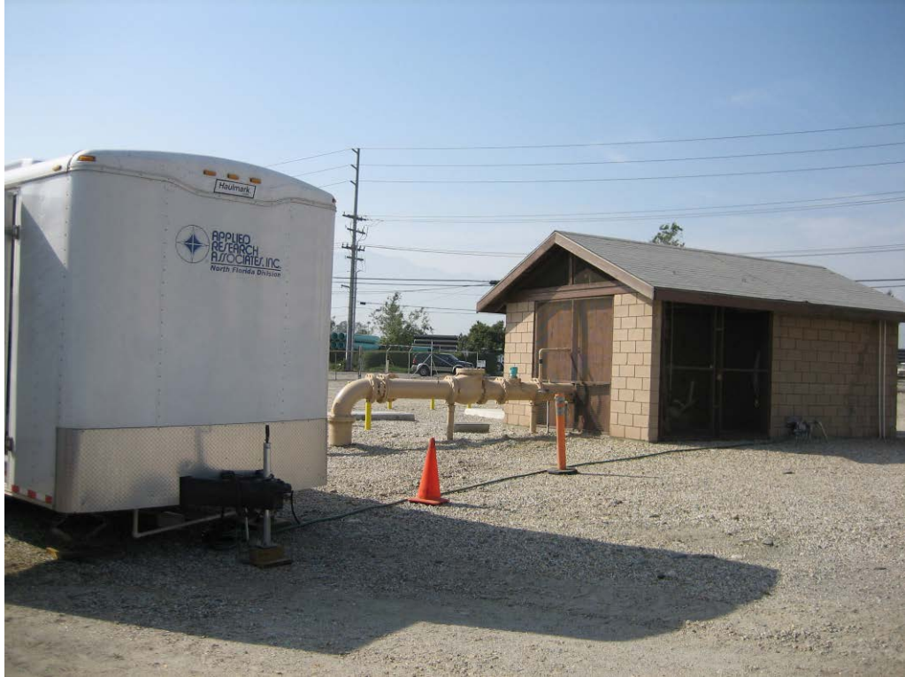
ARA demonstration trailer beside enclosure for well F-17C in Fontana, CA.
