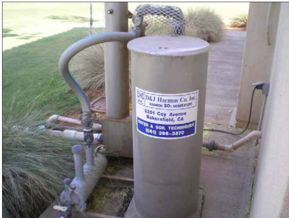
Photograph 14. Chemical mixing tank on subject property
