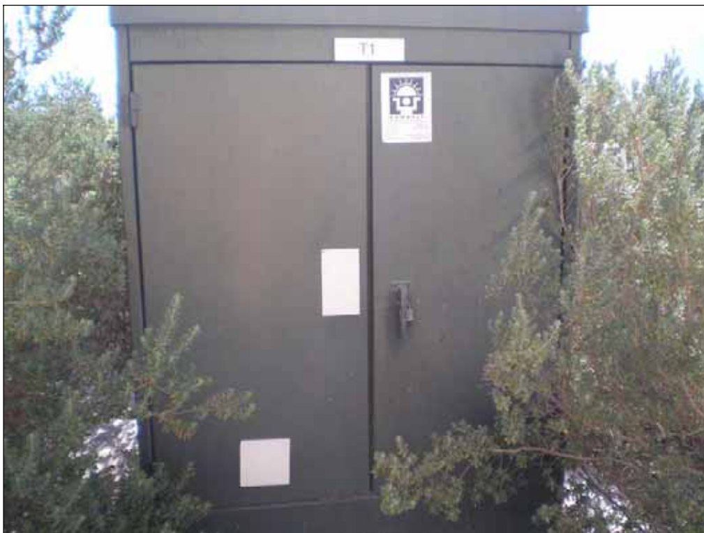
Photograph 12. Transformer on subject property
