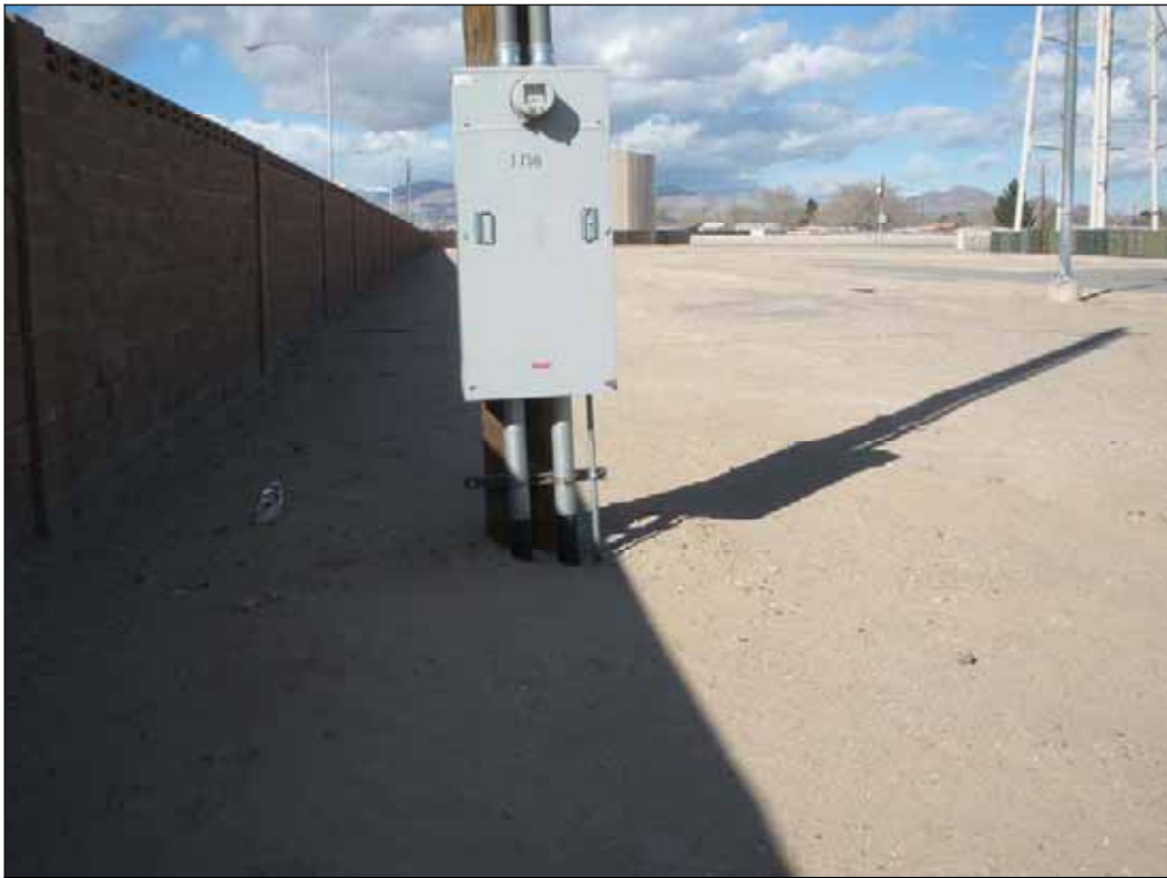
Photograph 16. Underground electrical service on subject property
