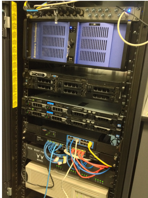
Figure 5. DEXTAR Servers, network switch and DVR.
