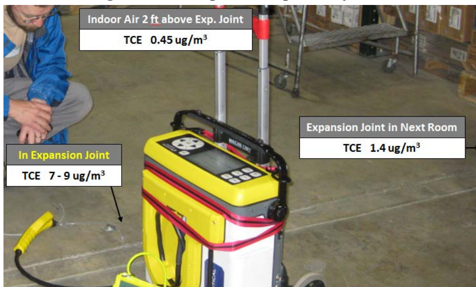
Figure 10: Example of a Vapor Entry Point
