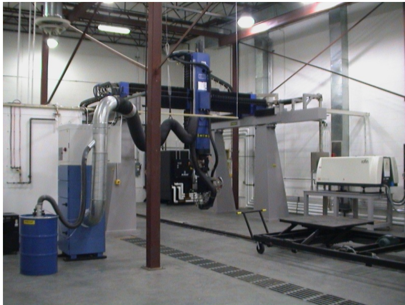
Figure 3. RLCRS installed at OC-ALC.
