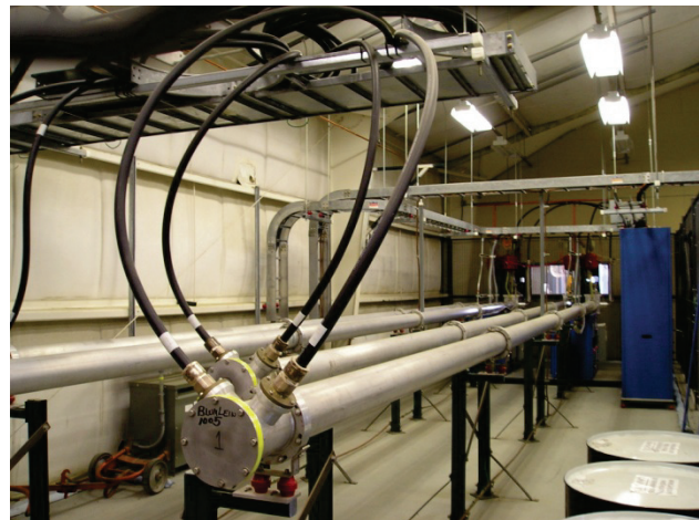
Figure 10. RHIC injection kicker Blumlein tri-axial pulse generators.
