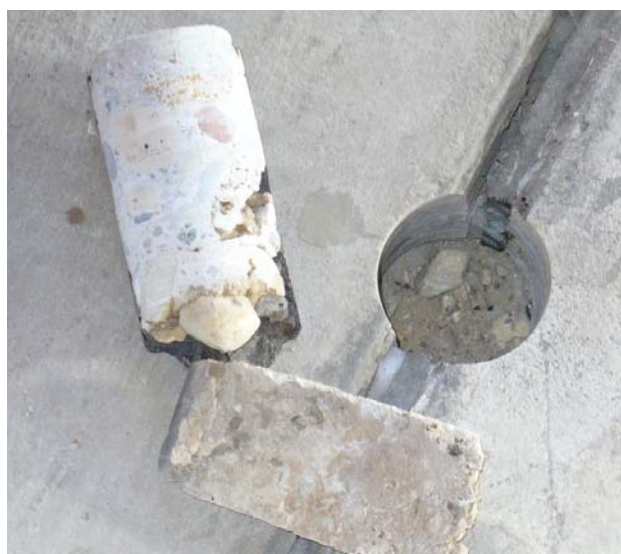
Figure 2-8 Core Taken at Expansion Joint
