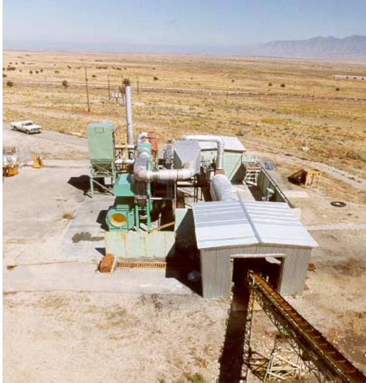
Figure 4. Production APE 1236 M1 Hazardous Waste Incinerator.
