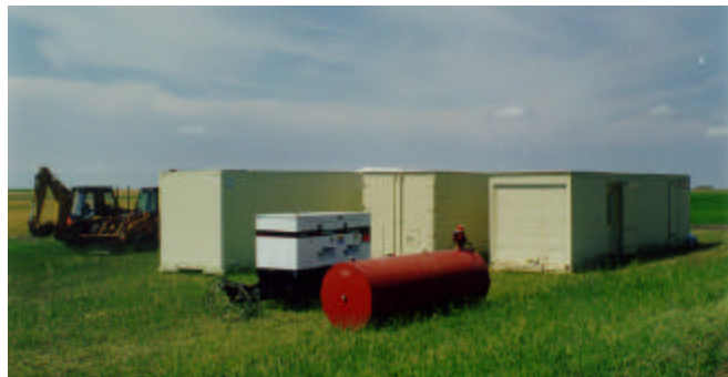
Figure 21. Base Camp for the survey showing the 3 support trailers, the backhoes, and the power generator
