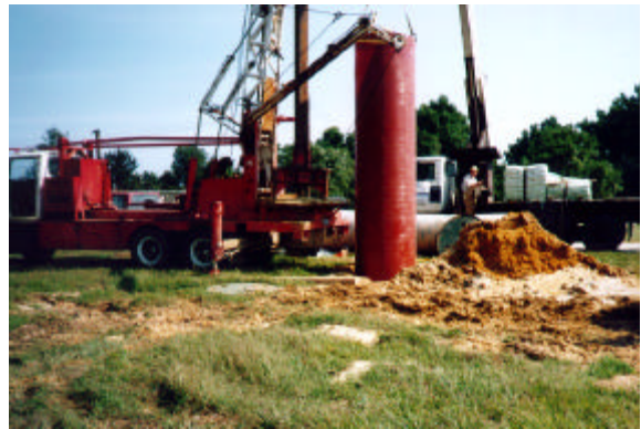
Figure 6. Fiberglass liner of the test well being lowered into place at CBD
