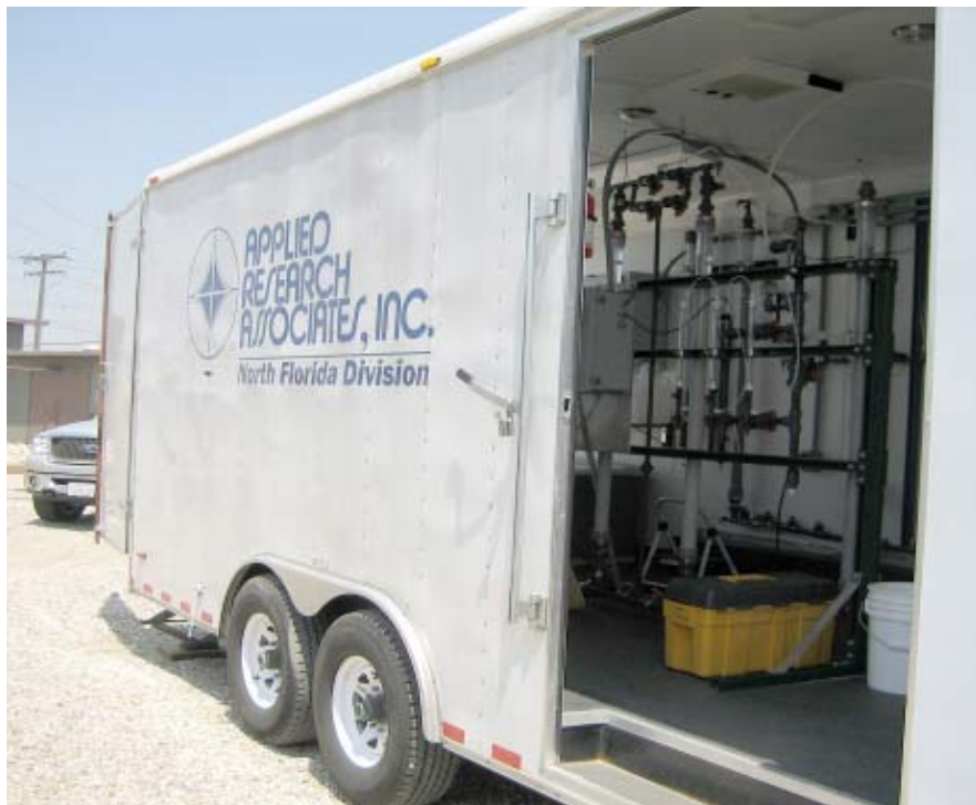
ARA Demonstration Trailer Containing Ion Exchange Equipment at Well-Site F-17 in Fontana, California.
