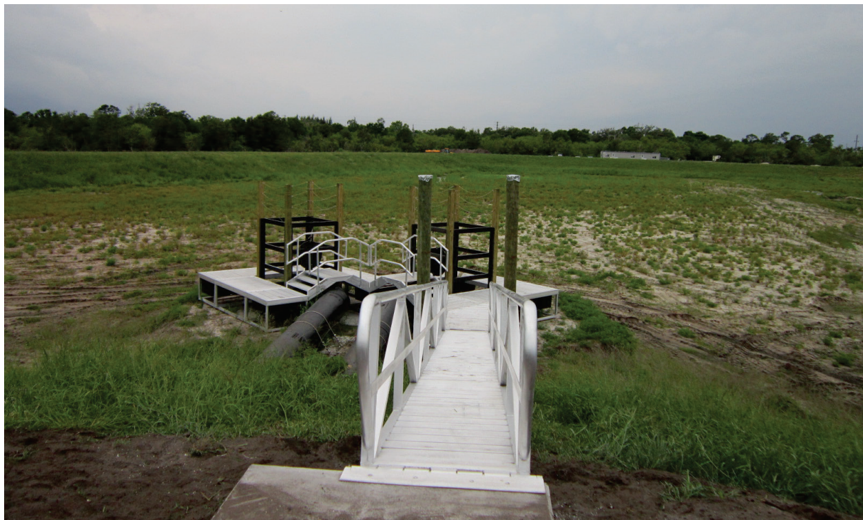
Figure 5. Set of 8.5-ft-tall, 5-ft x 5-ft box riser weirs with floating dock and gangway access, DMMA IR-2, Sebastian, Florida. Photo credit David May, Brance Diversified.
