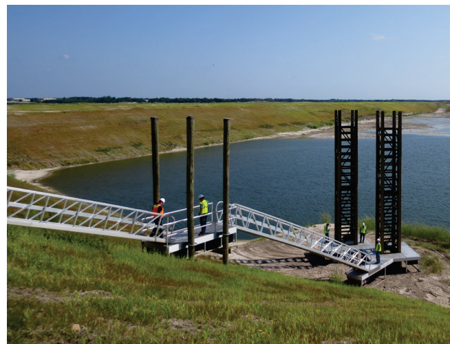
Figure 1. Set of 38-ft-tall, 4-ft x 4-ft box riser weirs (under construction) with dual-segment gangway to floating dock access, Bartram Island Cell B2, Jacksonville, Florida.
