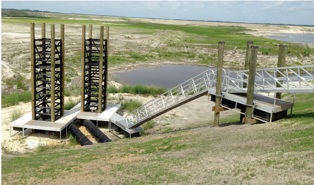
Figure 8. Set of 28-ft-tall, 5-ft x 5-ft box riser weirs (under construction) with dual-segment gangway to floating dock access, Bartram Island Cell A, Jacksonville, Florida. Photo credit Jose Bilbao.
