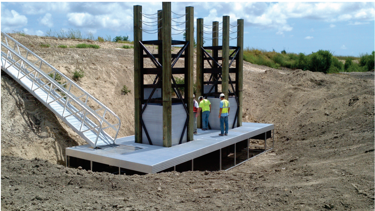
Figure 7. Set of 18-ft-tall, 4-ft x 4-ft box riser weirs with gangway to floating dock access, Bartram Island Cell F, Jacksonville, Florida.
