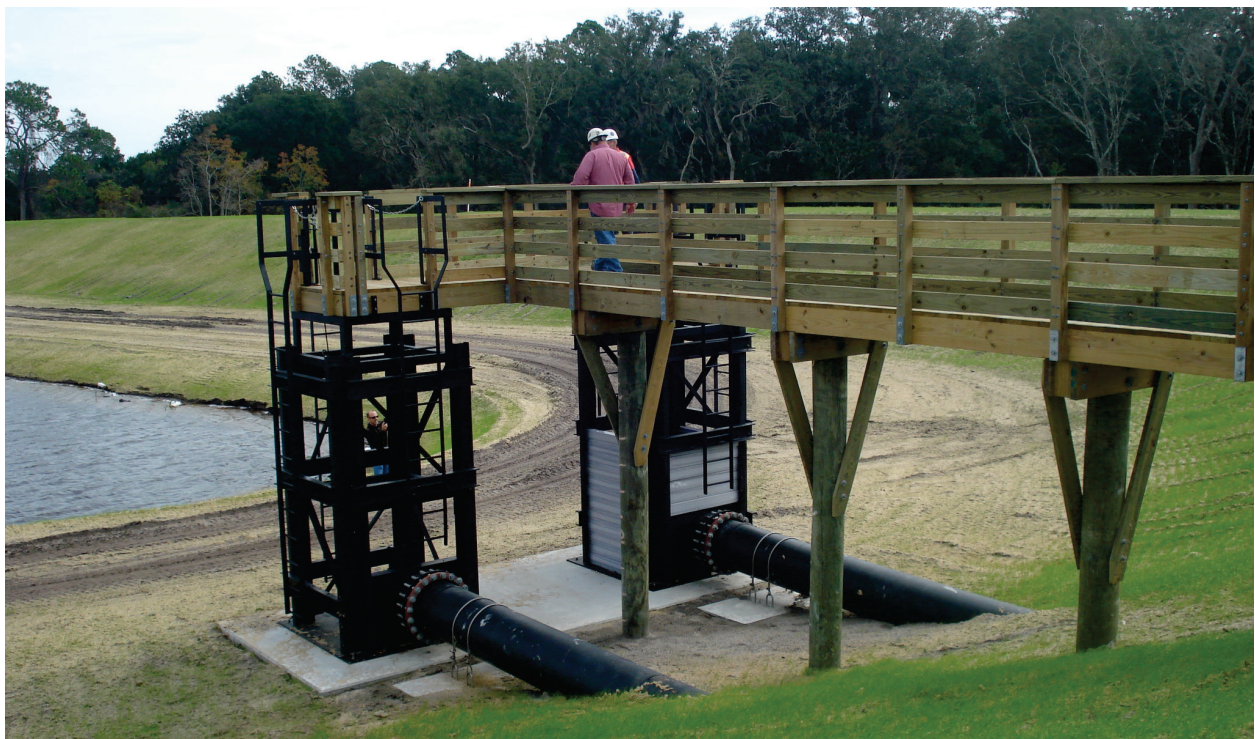
Figure 9. Florida Inland Navigation District site NA-1 designed by Taylor Engineering. Set of 11-ft-tall, 4-ft x 4-ft box riser weirs with gangway to floating dock access, DMMA NA-1, Fernandina, Florida. Photo credit Mr. Robert J. DiRienzo, Taylor Engineering.
