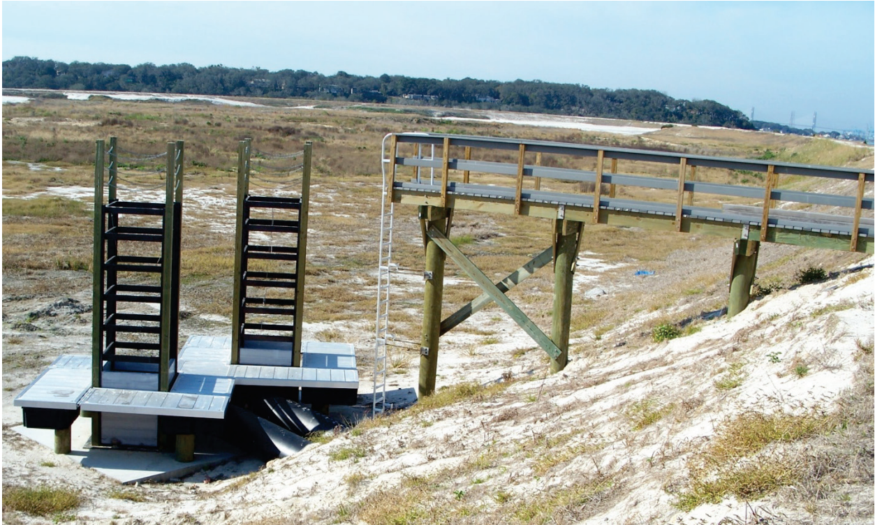
Figure 6. Set of 16-ft-tall, 4-ft x 4-ft box riser weirs with floating dock access, Buck Island, Jacksonville, Florida.
