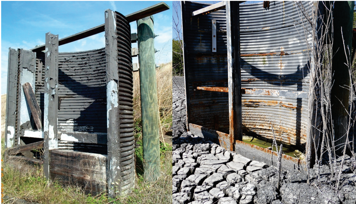
Figure 2. Historic half-pipe weir structure, consisting of a pile-supported corrugated riser and corrugated outfall pipes, with field-installed corrosion inhibiting coatings, Buck Island (right), Jacksonville, Florida and DMMA 2-D (left), Tampa, Florida.
