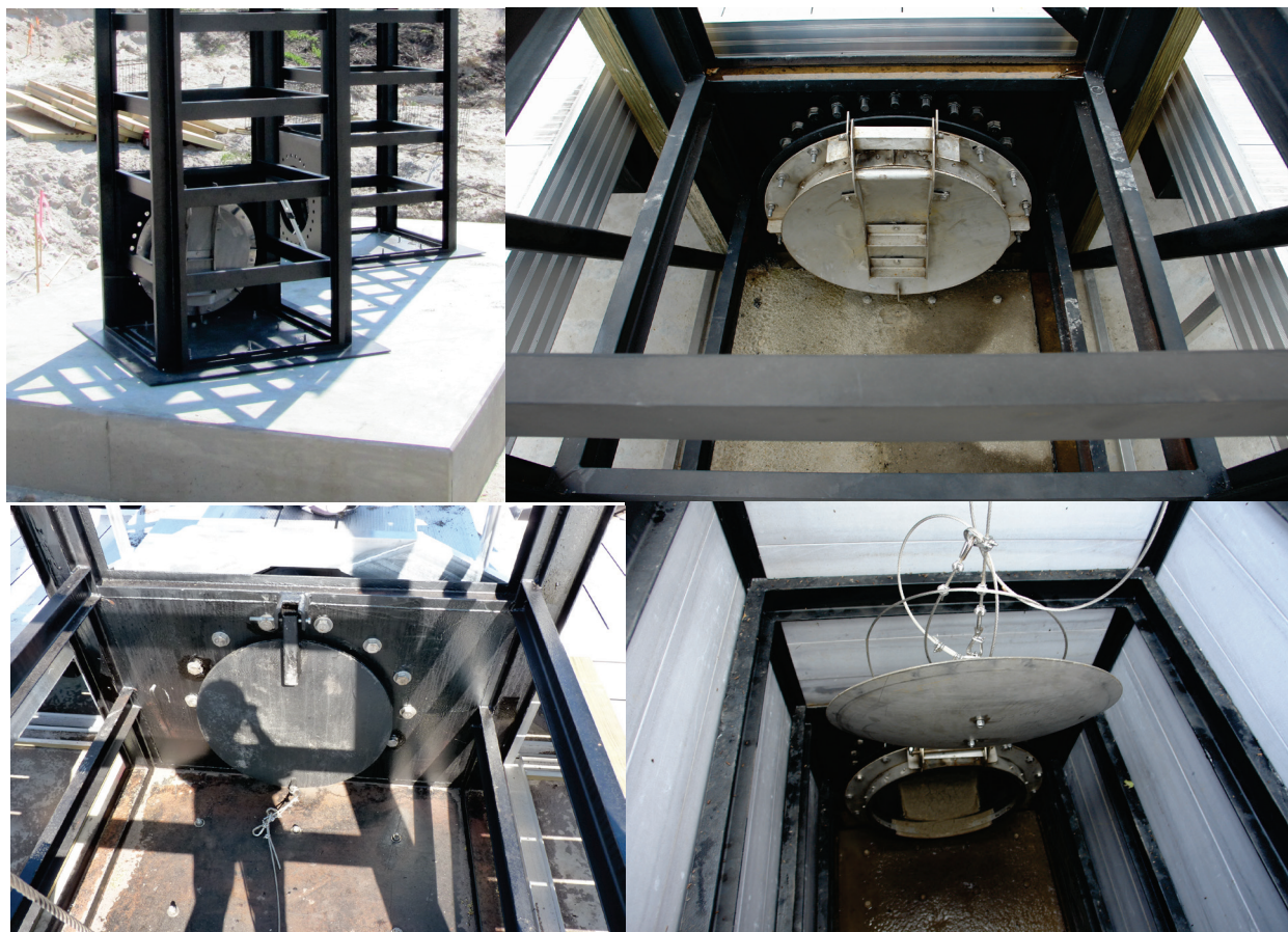
Figure 10. Internal weir outfall flap gates.
