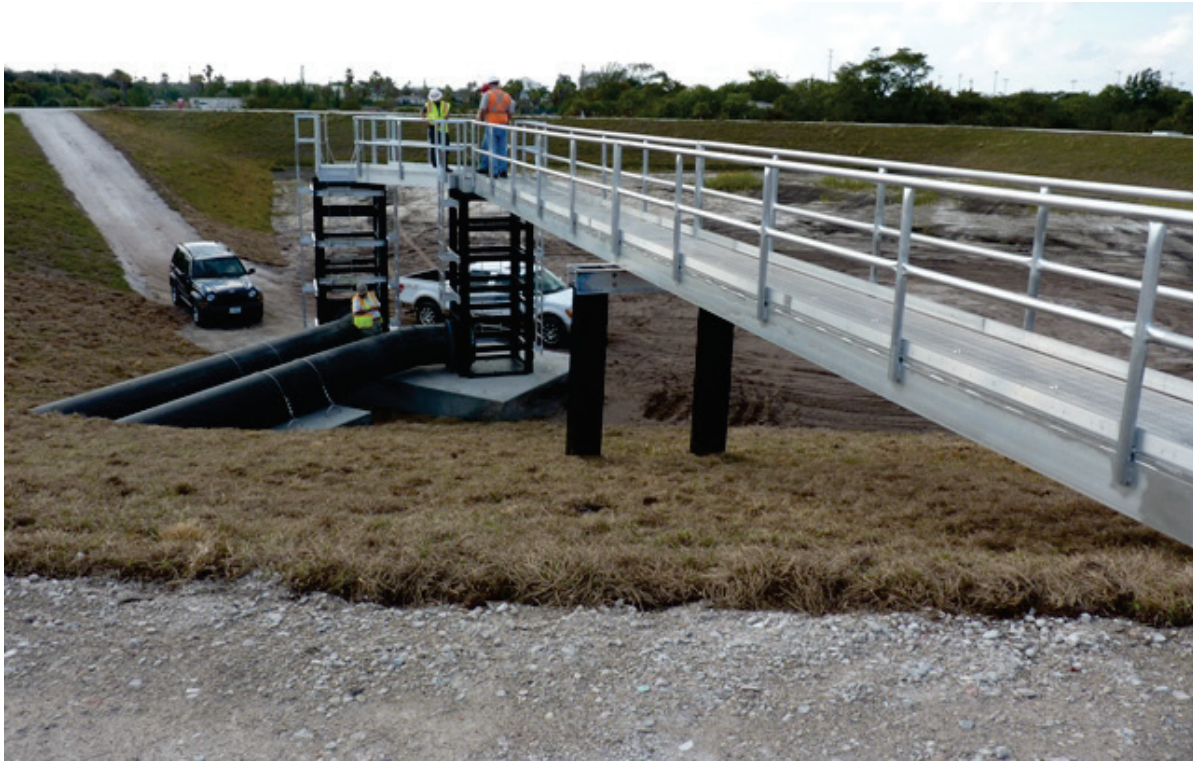
Figure 4. Set of 12-ft-tall, 4-ft x 4-ft box riser weirs with top access, MSA-641A, Delray Beach, Florida.
