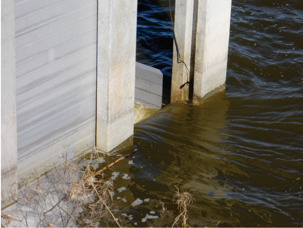
Figure 13. Composite weir boards in concrete box weir DMMA 2-D, Tampa Bay, Florida.
