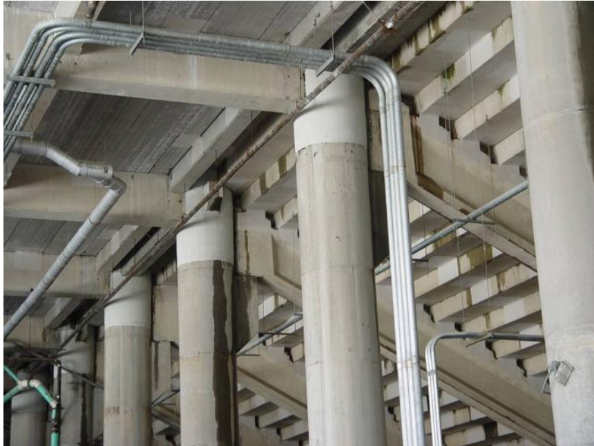
Figure 4. Composite wraps at column tops.
