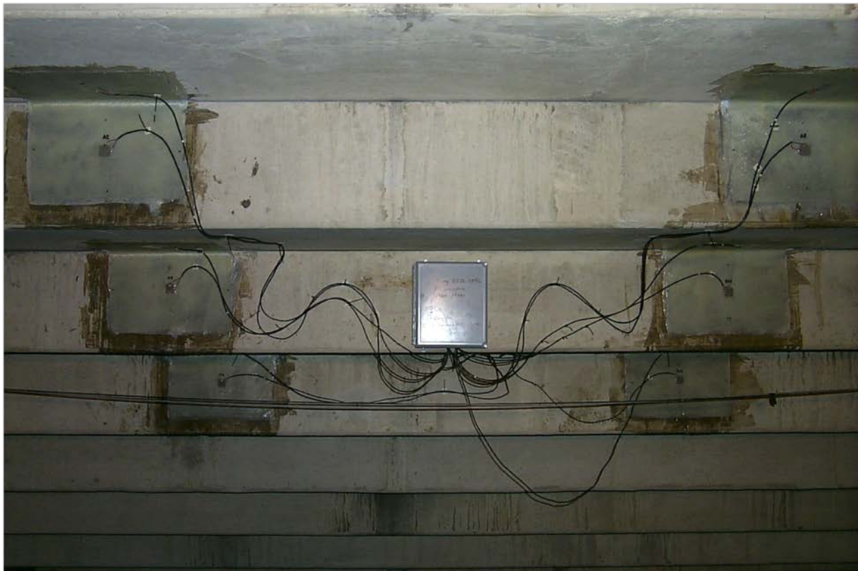
Figure 1. Structural support beams with FRP composite patches and piezoelectric sensors under Michie Stadium.
