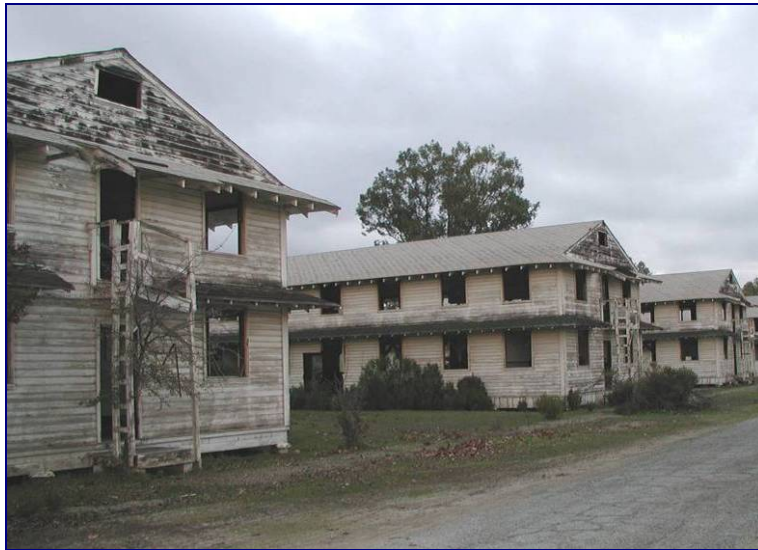
Figure 1.3. Vacant deteriorated WWII-era barracks coated with LBP.
