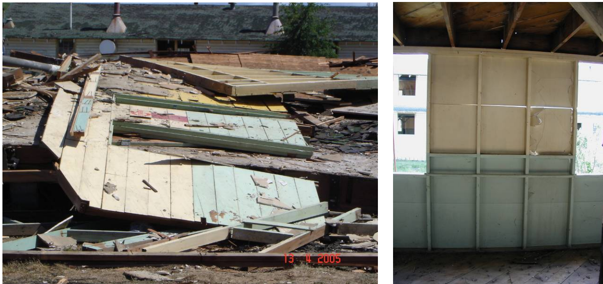
Figure 4.17. LBP-contaminated interior wall boards (left) and exterior wall studs (right) destined for landfill.
