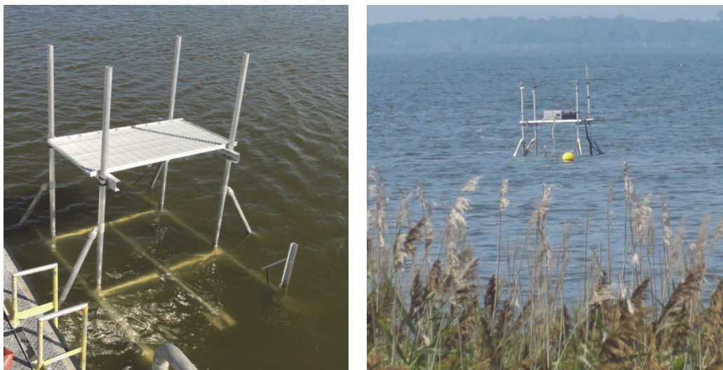
Figure 8. Instrument platform in Currituck Sound. Close-up of the platform during construction is shown on the left. A view of the platform from the shore is shown on the right after instrumentation was mounted to the platform.
