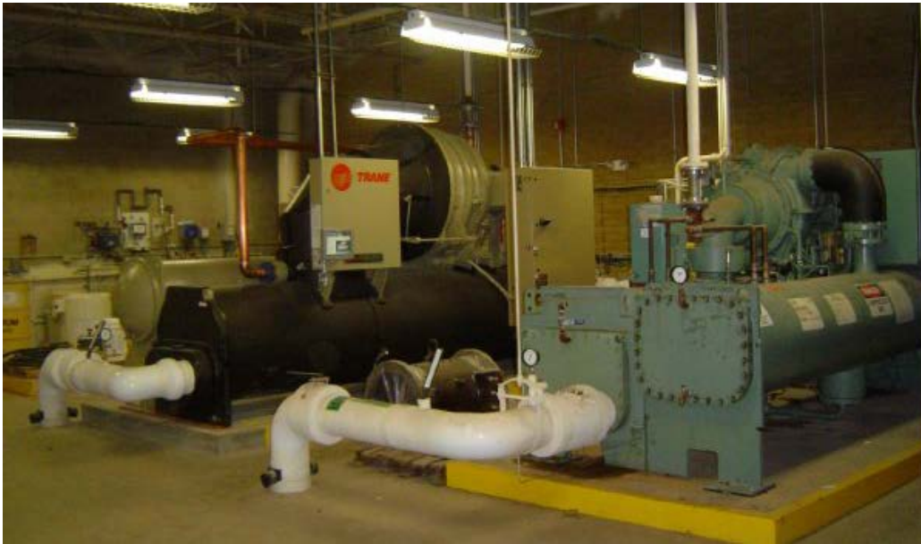
Figure 4. Chillers at Fort Huachuca SCP, showing Zeta Rod components mounted on wall in background.
