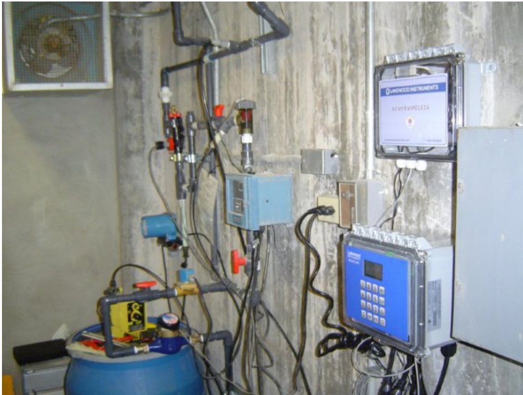
Figure 16. Fort Irwin Building 263 (control) monitoring components.
