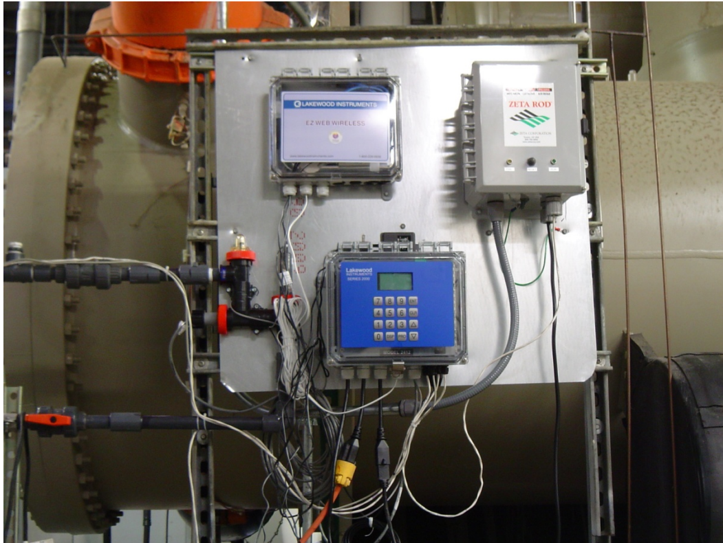
Figure 22. Water-management system components.
