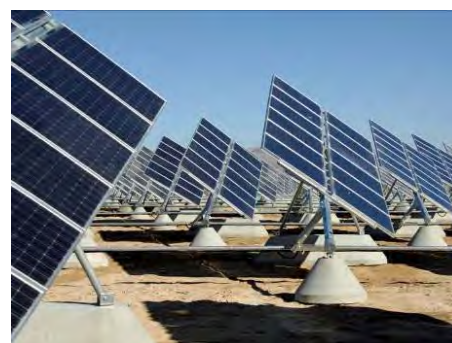
Completed solar power system with single-axis tracking arrays.
