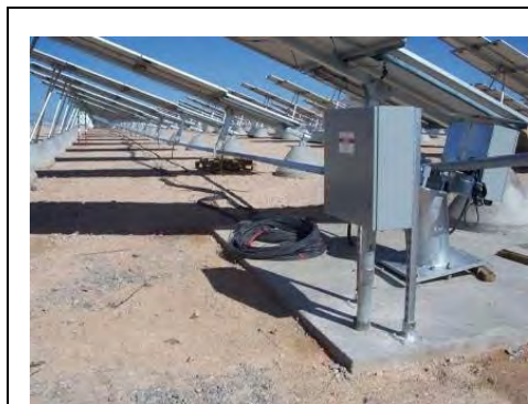
Concrete footings of the solar panels.
