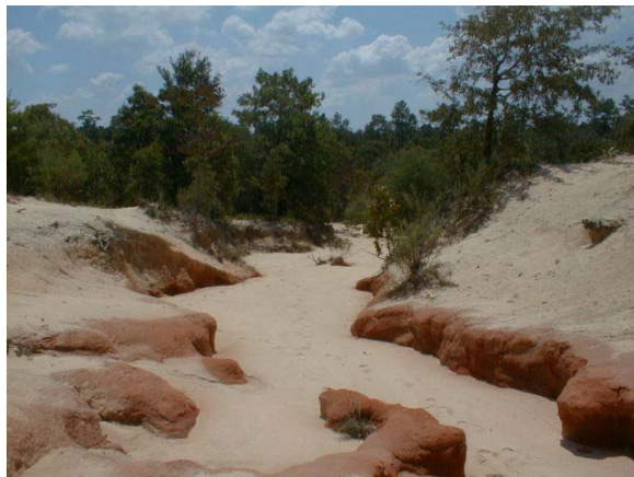
3-44a. Gully along the southern edge of TT-3 that has been incised and again filled with sediment
