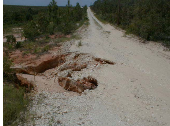
3-42f. Eroded road surface caused by the accumulation of road down gradient water flows
