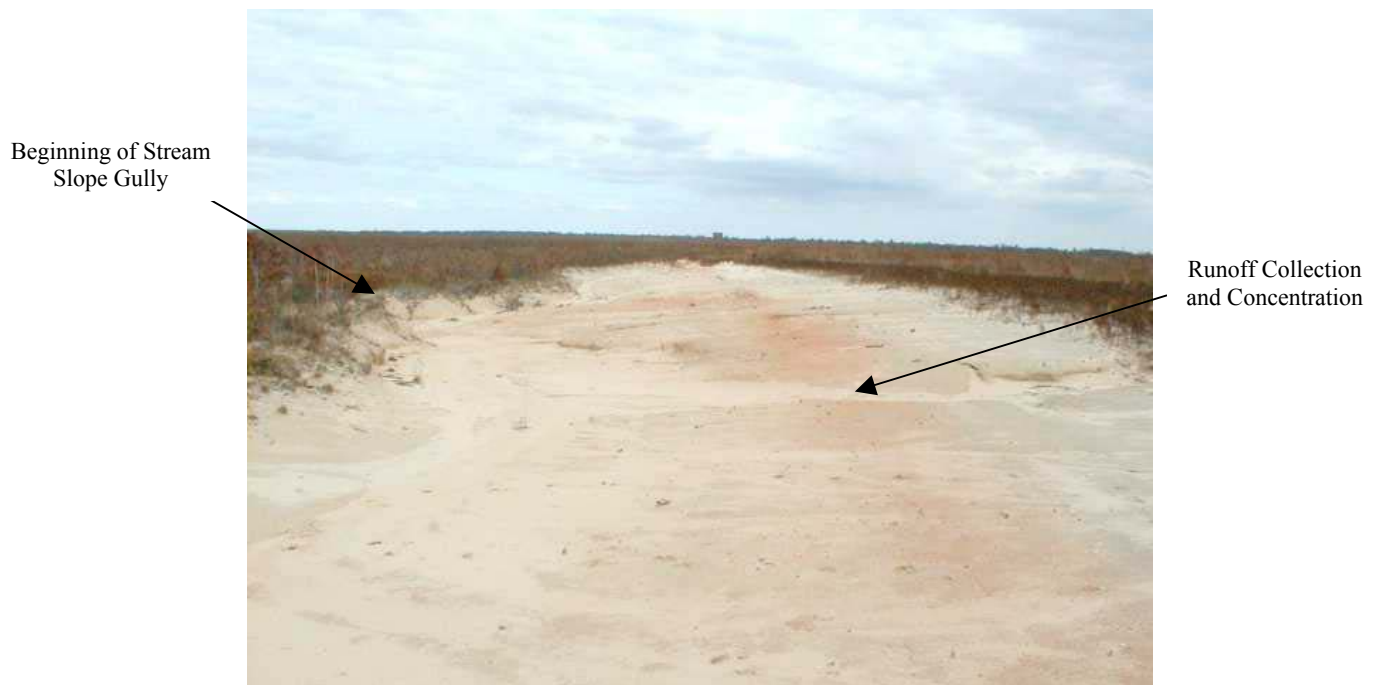
Figure 3-39. Primary Oakie Creek Ridge Road Erosion Site
