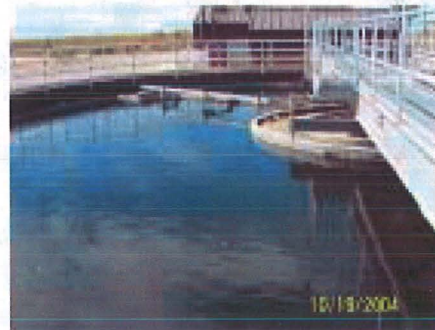
Photograph 4: View of the southern secondary clarifier at the wastewater treatment plant.
