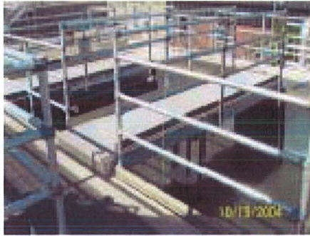
Photograph 1: View of the grit removal system at the wastewater treatment plant.
