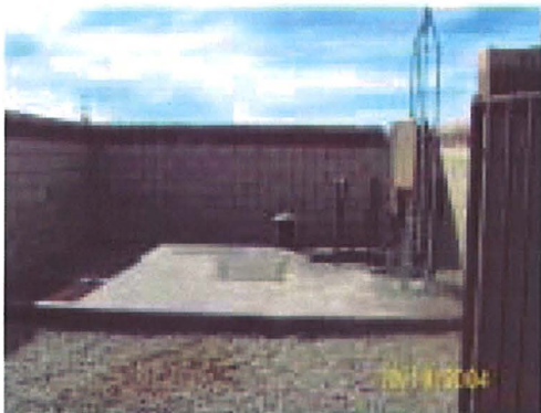
Photograph 9: View of a typical lift station (specifically, Lift Station 25) at HAFB.
