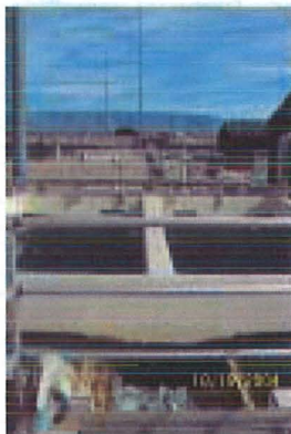
Photograph 5: View of the dechlorination basin at the wastewater treatment plant.
