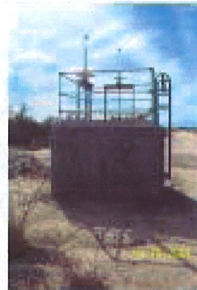
Photograph 10: View of the splitter box located southeast of the wastewater treatment plant.
