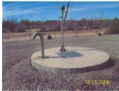
Photograph 8: View of Lift Station 23, located at the wastewater treatment plant.
