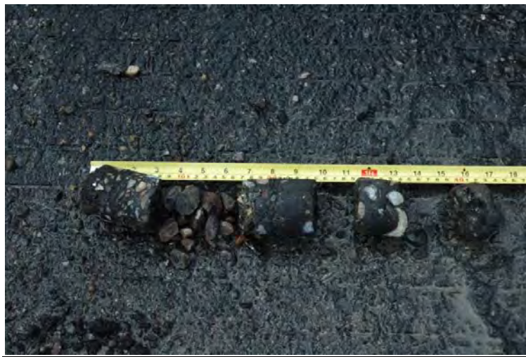
Figure 2-1 Asphalt Pavement Core – Runway 17-35 Core No. 2 (July, 2009)
