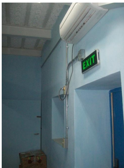
Figure 44. Use of surface-mounted electrical conduit.
