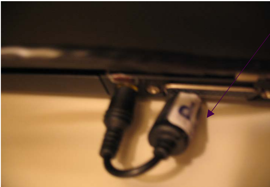
Server Power Cable from Server to Outlet
