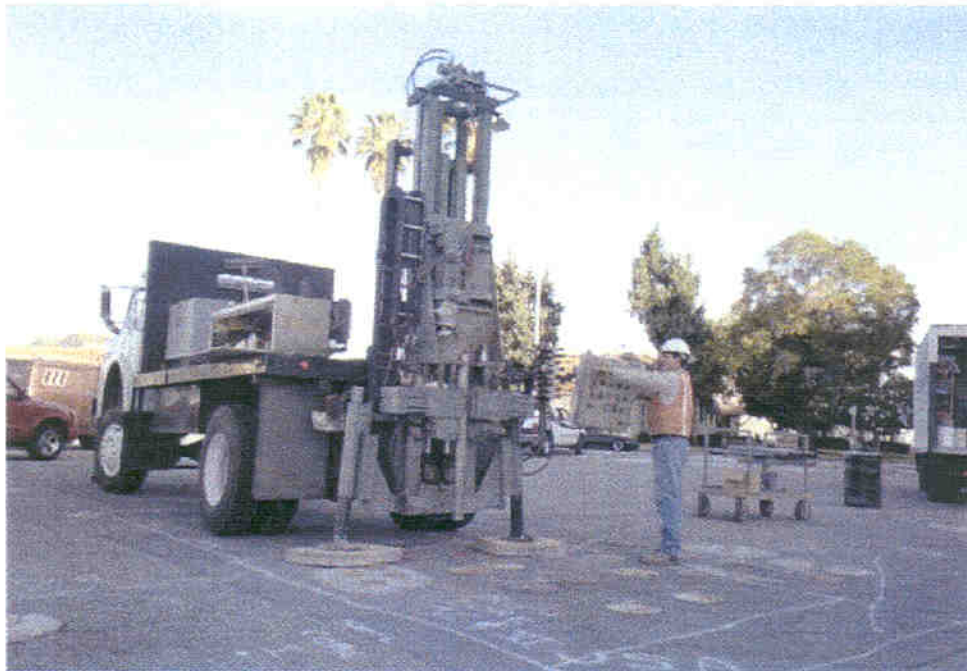
Figure 4-3. Rig used to collect iron core samples from the former NAS Moffett Field PRB.
