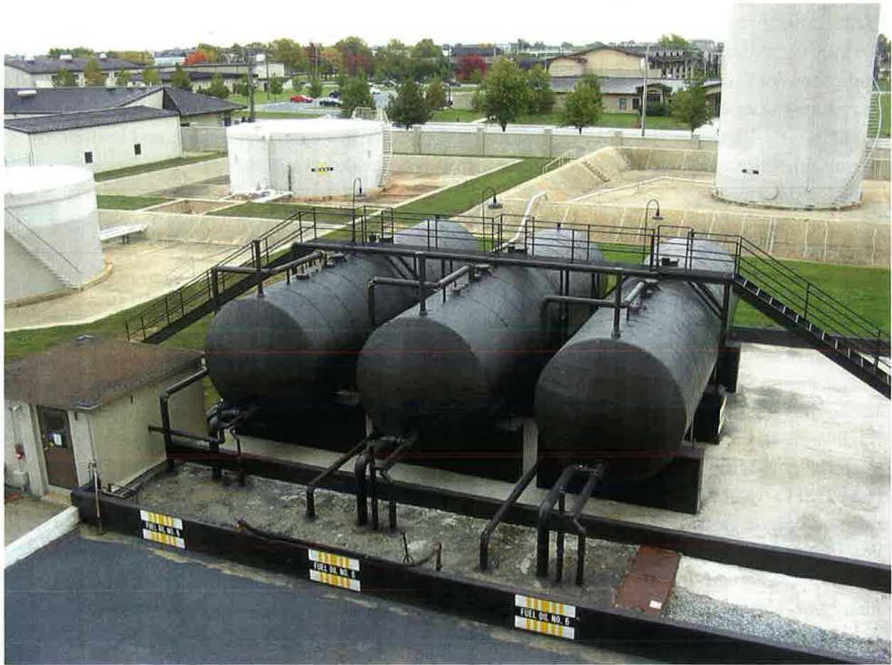
Figure 3.4-1. Aboveground Storage Tanks at Central Heat Plant
