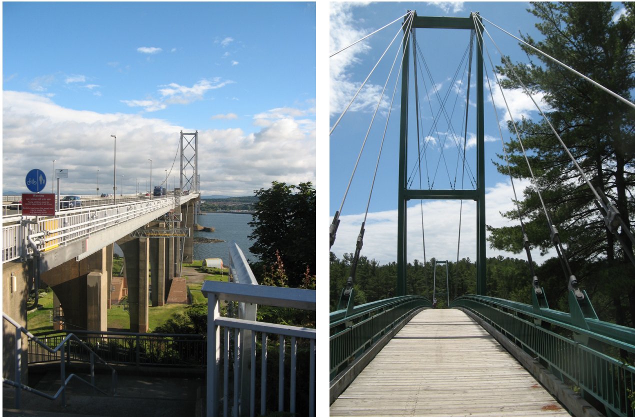
Figure C-19: Two Contrasting Suspension Bridges. (a, left) The Forth Road Bridge that carries expressway traffic across the Forth River, Scotland; (b, right) A bridge across the French River, Ontario, Canada, designed for snowmobiles and pedestrians, though capable of supporting a car (Photos by the Author).
