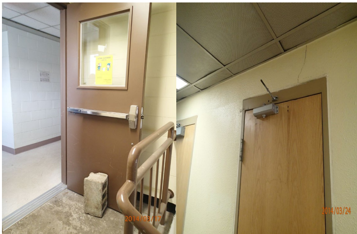
Figure 4. Ineffective use of fire doors allows fire to draft through the entire building. Left: Fire rated doors often propped open (Deficiency No. CAS-FP-140317-024) Right: Broken automatic closing mechanisms (Deficiency No. CRC-FP-140324-013) Source: DoD OIG
