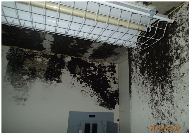
Figure 10. Mold unchecked, unreported, and unmitigated (Deficiency No. OSA-EN-140407-007) Source: DoD OIG
