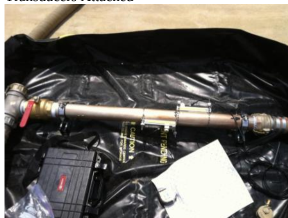
Figure 5.3.11 Flow Pipe with Ultrasonic Transducers Attached
