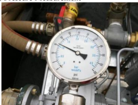
Figure 5.3.9 Pump Discharge Pressure Measurement
