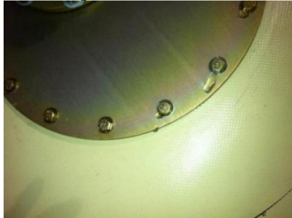
Figure 4.5.23 – Manway / Filler / Discharge Bolt Leaks
