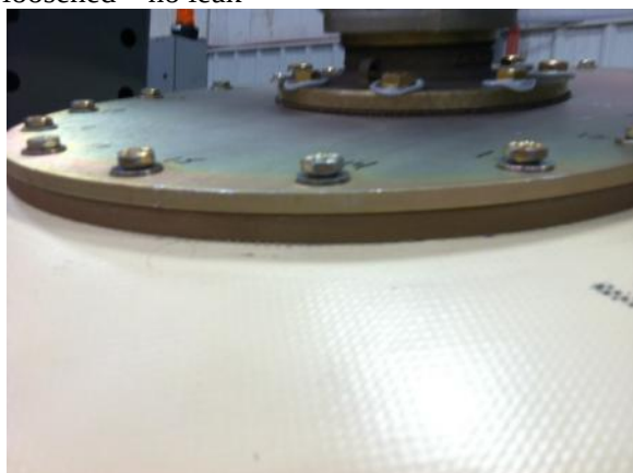
Figure 6.2.101 – Tank fitting with bolts 12-15 loosened – no leak
