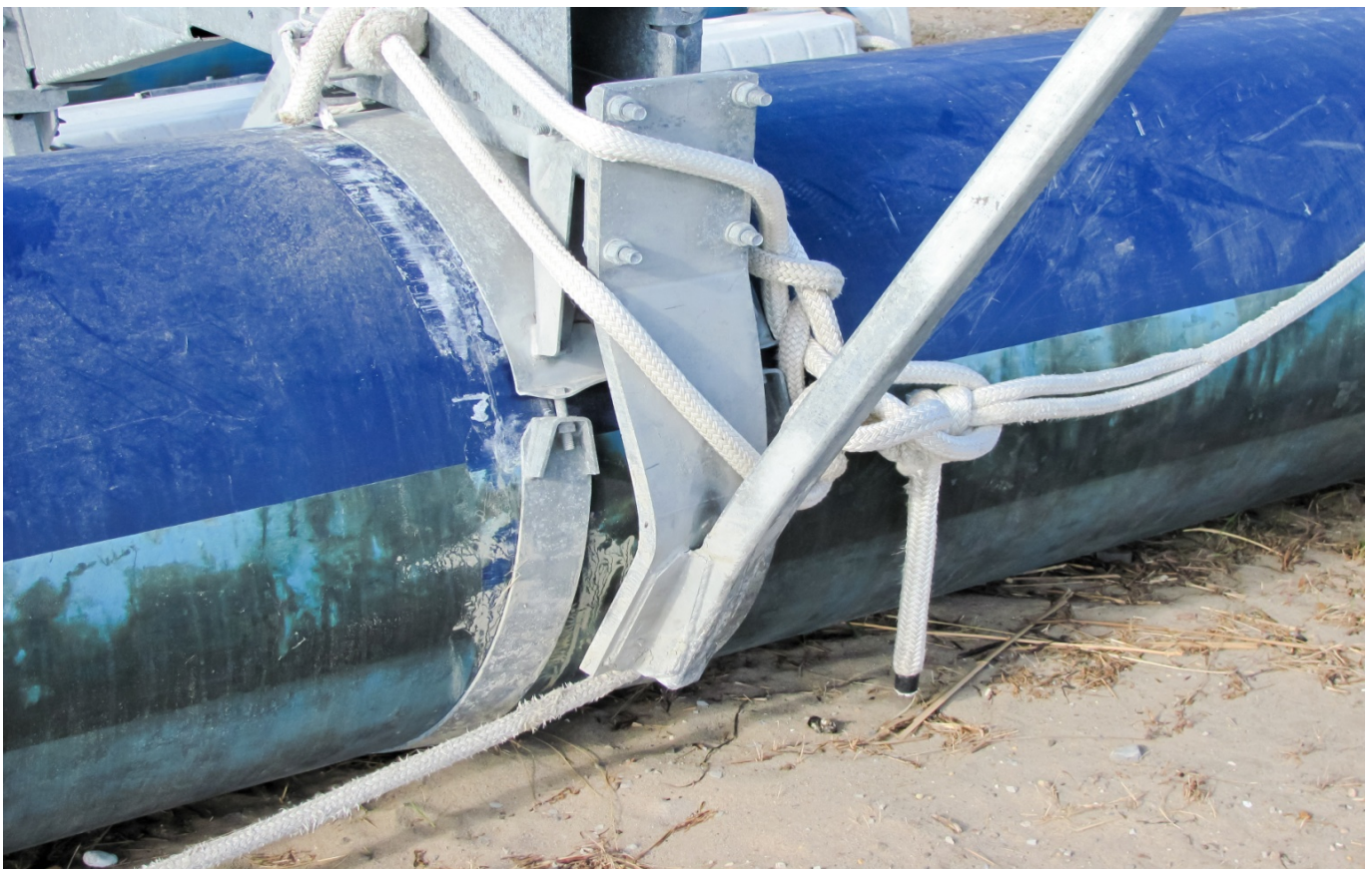
Figure B-1. Damaged guide and belly band.
