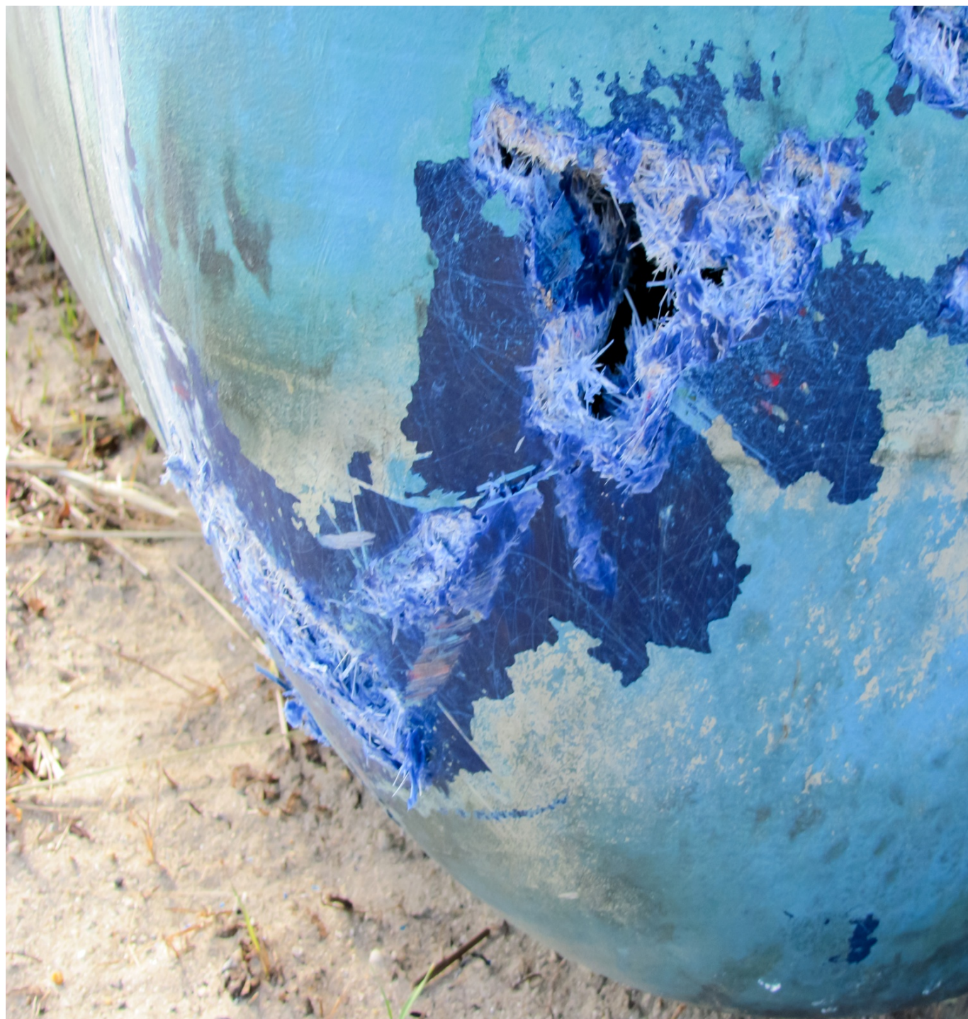
Figure B-2. Damaged area of pontoon.
