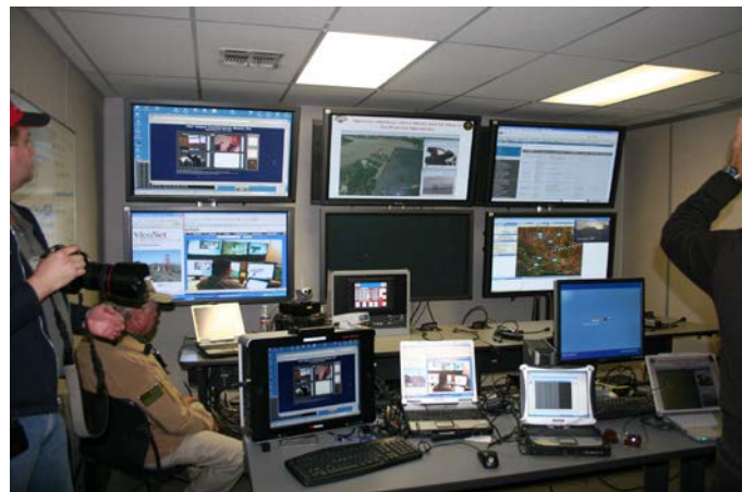
Figure 11. TNT Technical Operations Center (TOC)
