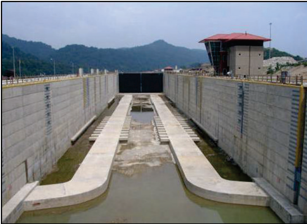
Figure 4. Dry bed view of the Marmet Lock in-chamber longitudinal culvert system, looking downstream.
