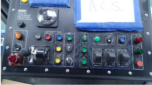
Aft Control Station Markey Control Panel
