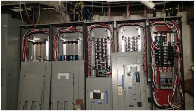
Upper MMR Power Panels
