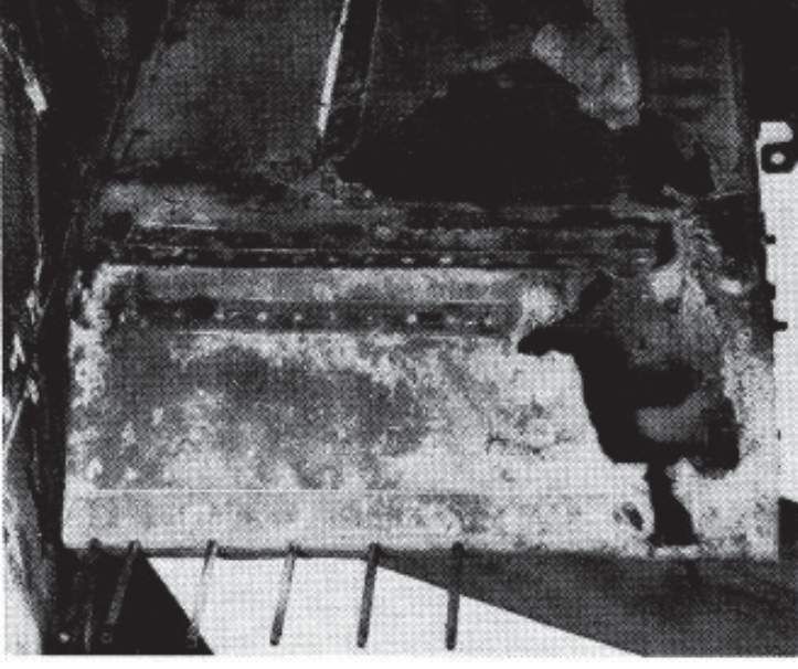
Shock impingement damage to support fin
