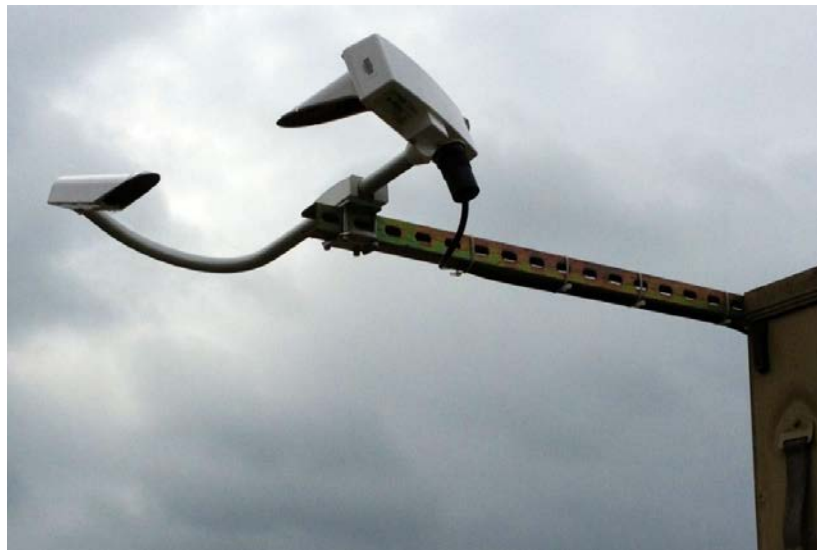
Figure 12. Visiometer deployed on the shelter.
