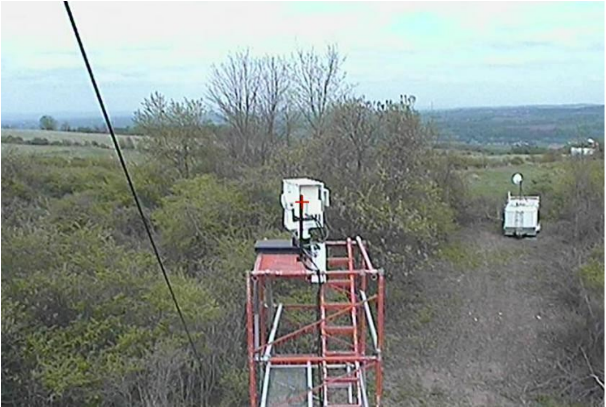
Figure 29. Optical terminal and Rapidlink antenna at Stockbridge
