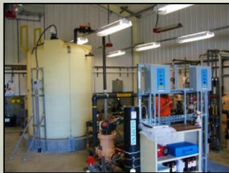
Class A Recycled Water Plant
