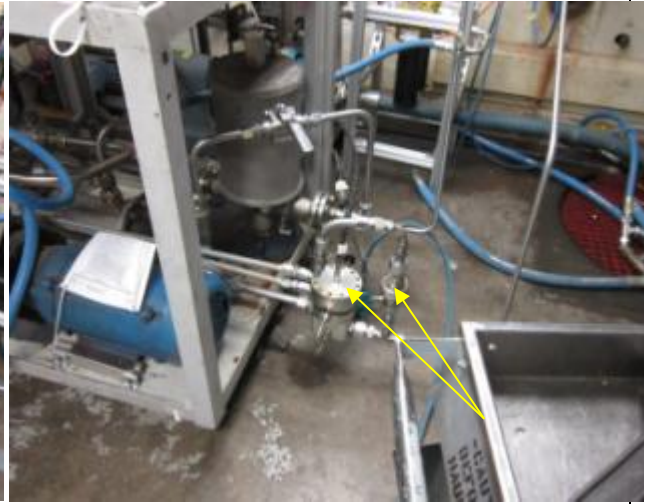
Pressure control valve and burst disk
