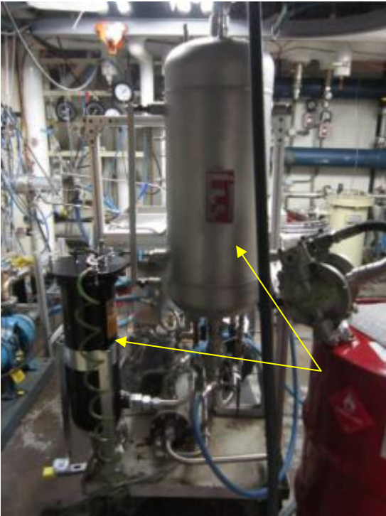
Low Lube Set Up: Supply Tank & Clay Filter (on left)
