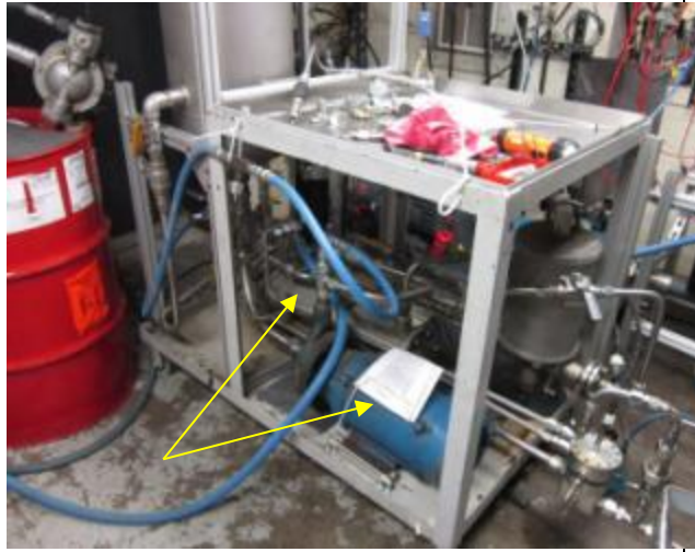
Heat exchanger and boost pump
